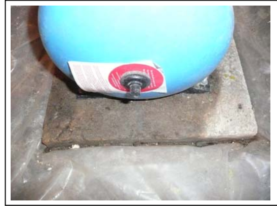
Photo 2. The darker area indicates moisture adsorbed from the air in the crawlspace into the concrete block. The concrete is cooled by the ground and the relative humidity of the air in contact with the concrete increases as it is cooled, driving the adsorption and absorption processes.
