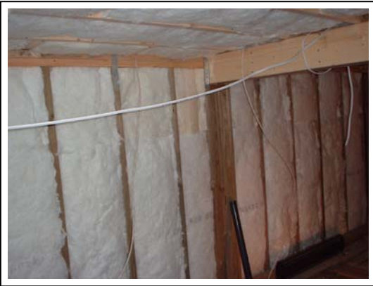
Photo 1. Exposed ground in a crawlspace is typically several degrees cooler than the crawlspace ambient air temperature. The bottom edges of floor joists exposed to the ground are typically within a few degrees of the ground surface temperature due to radiation dominated heat transfer. At these locations, the relative humidity is higher and the moisture content of the wood is elevated.
