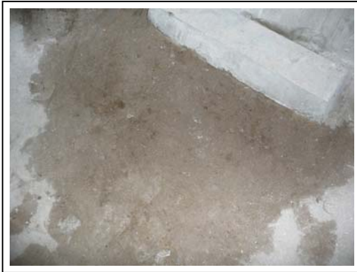
Photo 1. Wet crawlspace ground indicates wicking of moisture through the sand. Poor drainage caused rain water to flow towards the building and then seep down and under the foundation walls. Exposed, wetted materials provide a source of moisture.
