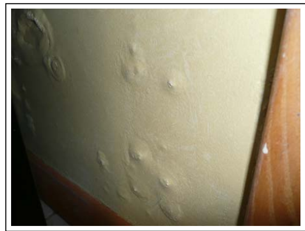
Photo 3. Snow melting in the adjacent space absorbed into the concrete slab on grade, moved laterally to below the bottom wall plate and then upward into the wall assembly where it caused blistering of the wall finish.
