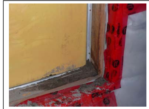
Photo 2. A roof drain leader discharging adjacent to the crawlspace wall resulted in water and sand entering the crawlspace through the gap between the crawlspace door panel and jamb. Entering water pooled on the ground cover material, providing a source of moisture.
